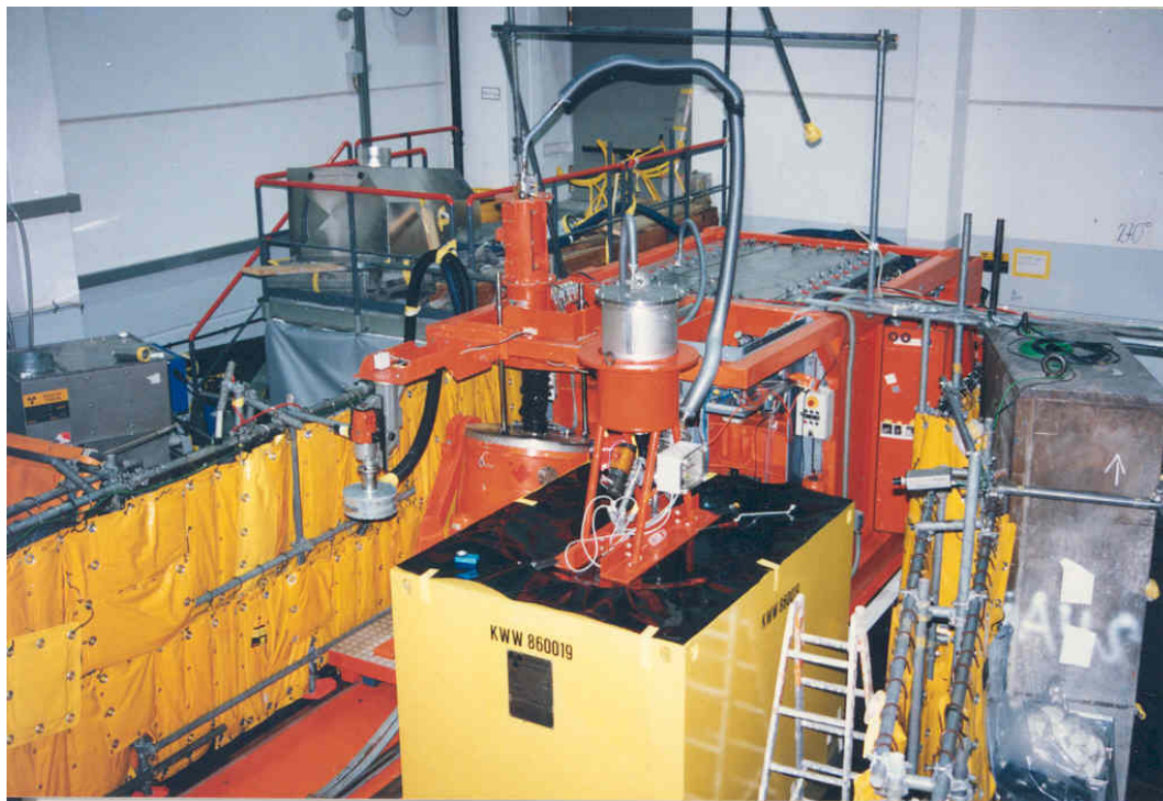
Fig. 4. Overview over the treatment unit
