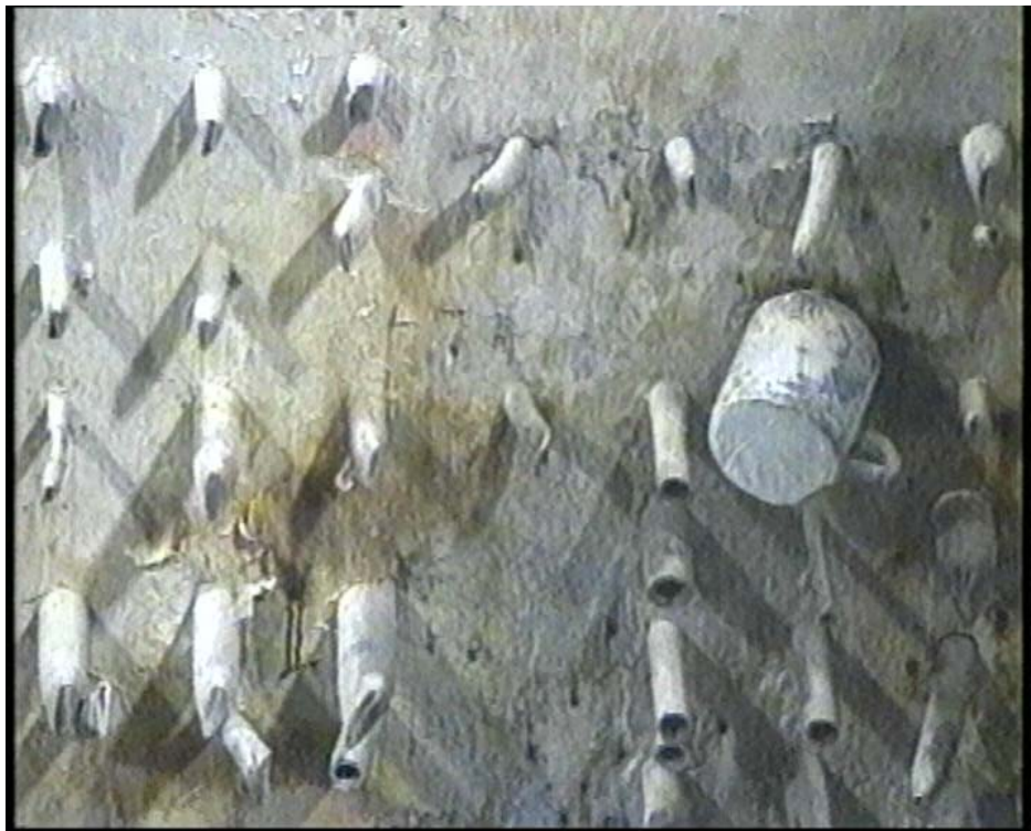
Fig. 3. Partly open ducts with additional shielding
