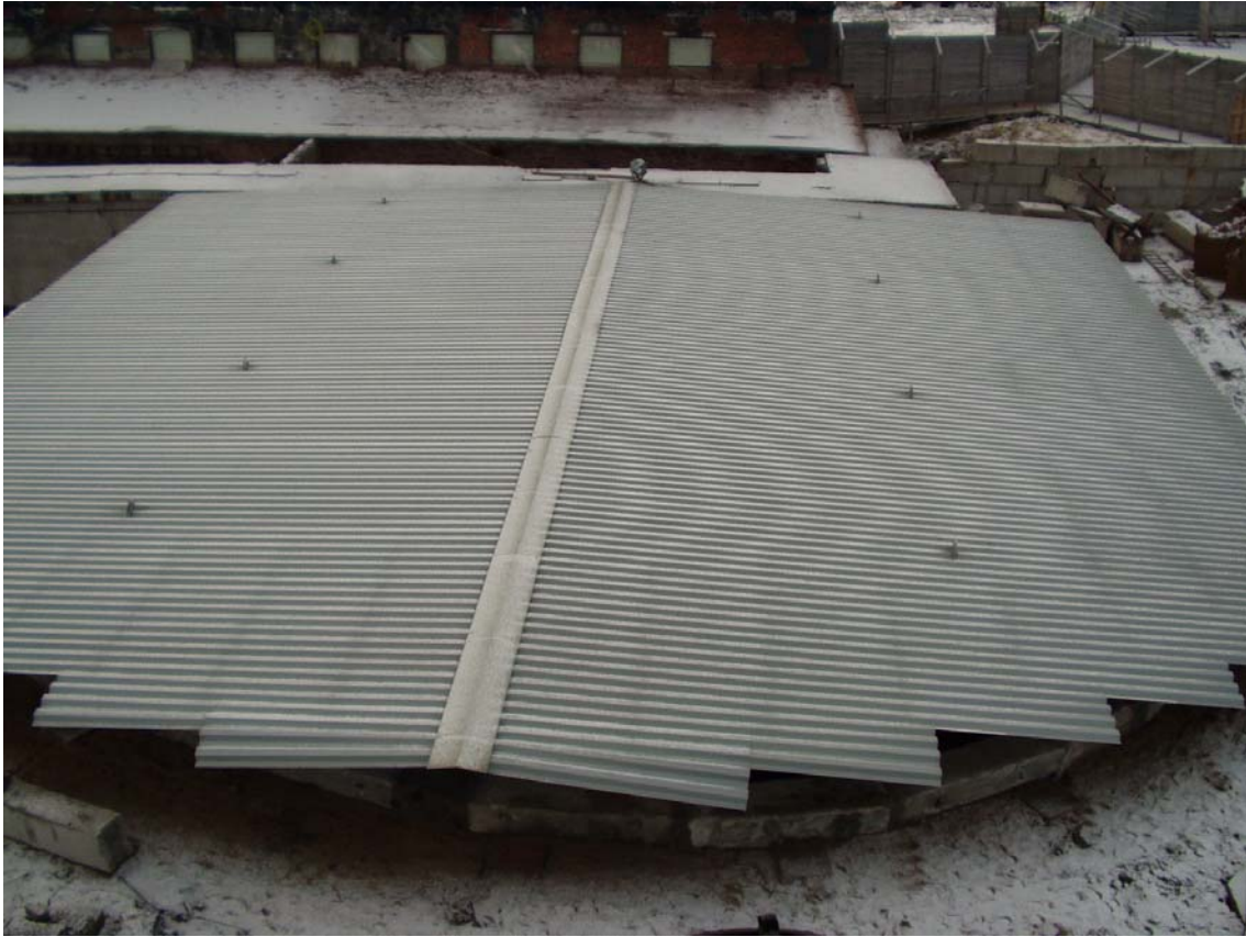
Fig. 2. Temporary cover installed over dry storage Unit 1 (facility 3A)
