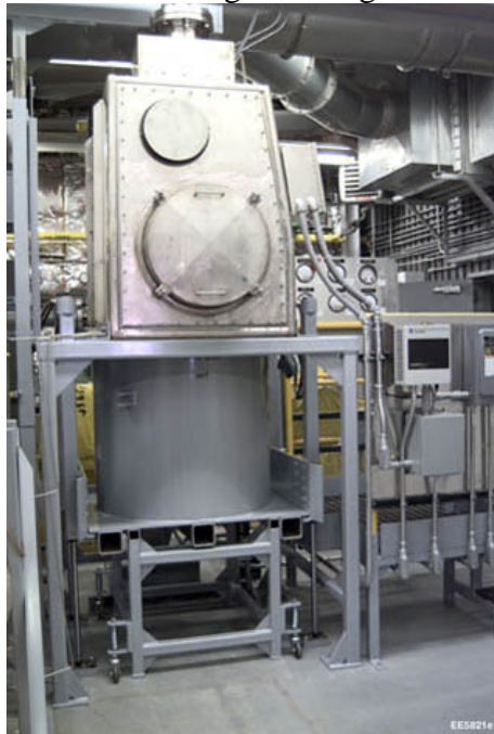
Fig. 3. SCMS Solidification Station Shielded Over Pack.
