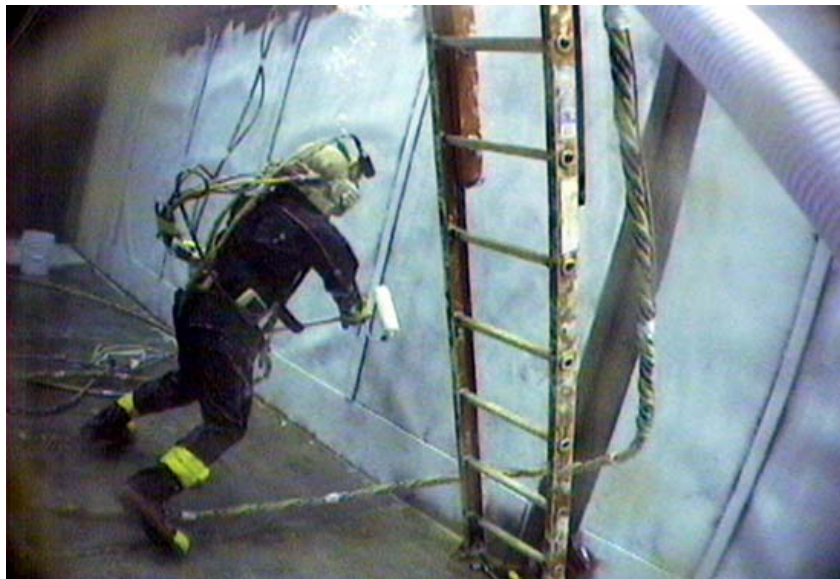
Fig. 3. Divers apply a two part epoxy fixative underwater to eliminate airborne contamination.
