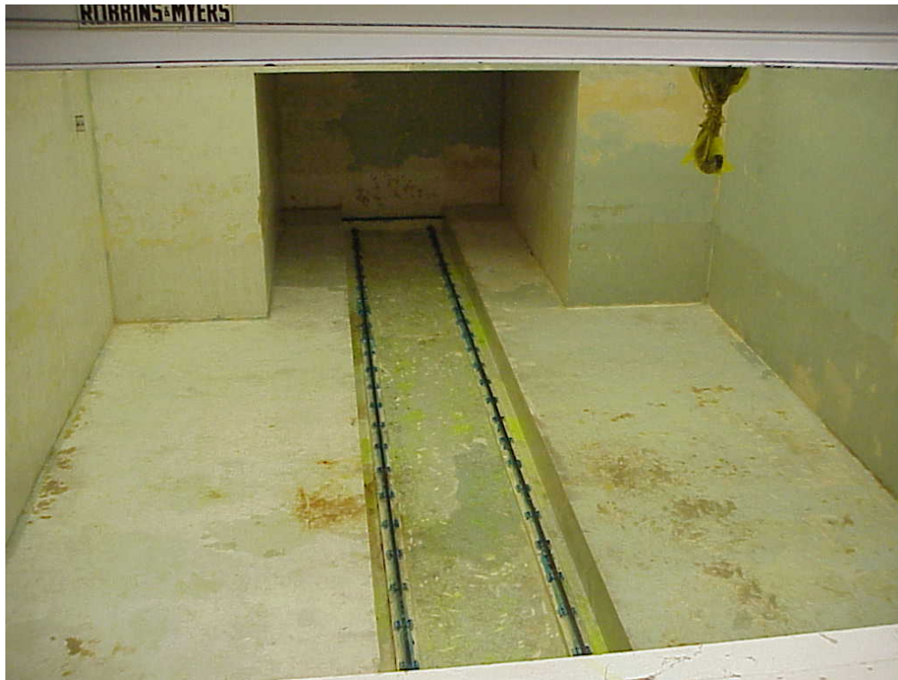
Fig. 4. Test Area North spent fuel basin with fixative applied and water removed.
