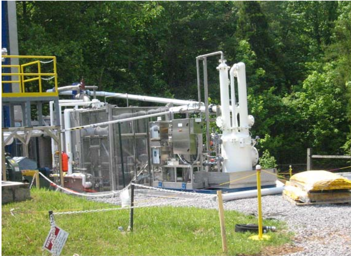
Fig. 3. Scrubber module (photograph taken in Oak Ridge).
