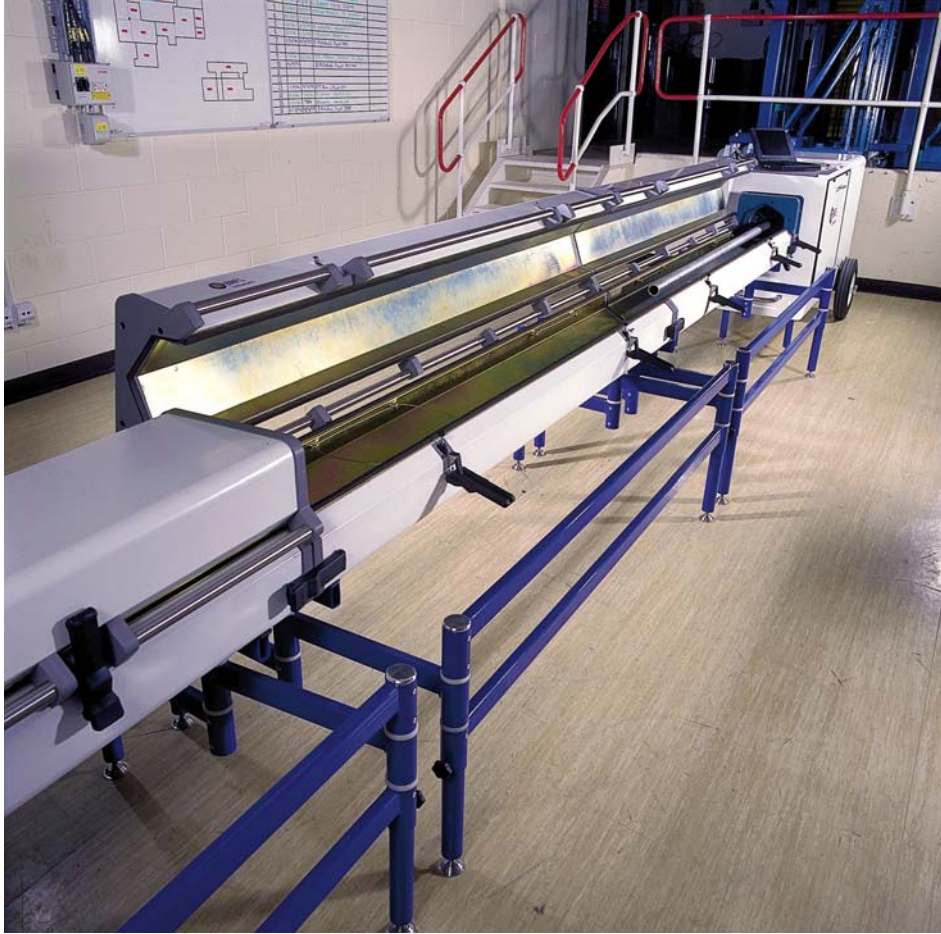
Fig. 2. Pipe monitor at the BNFL Sellafield Nuclear Facility
