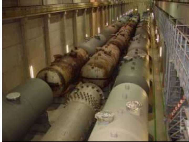
Fig. 1. Blocked place through steam generators and pressurizers in interim storage
