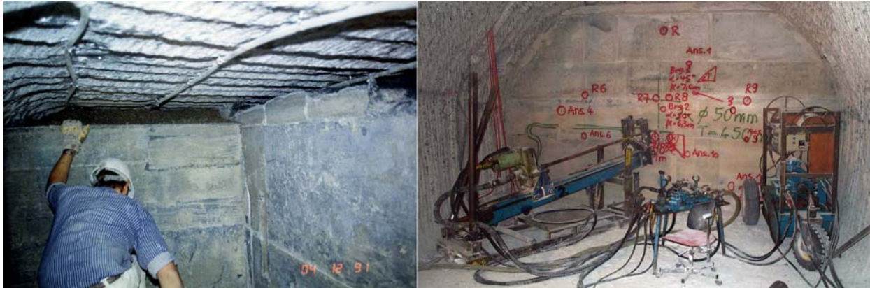
Fig. 1. Construction phase of the salt-concrete Asse seal showing salt-concrete segments, the partly filled gap and the injection pipes (left) and start of the investigation program (right).
