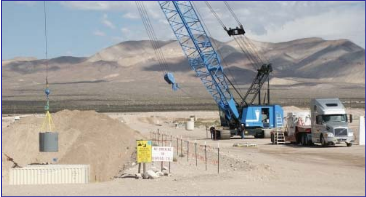
Fig. 3. High-activity low-level radioactive waste monolith from Foster-Wheeler is positioned for disposal in cell 11 at the Area 5 Radioactive Waste Management Site.
