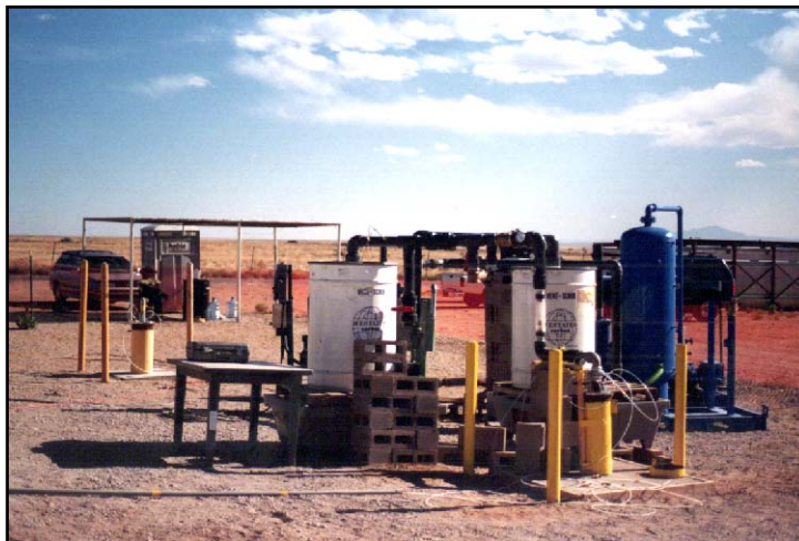
Fig. 1. Pilot Testing of Active Vapor Extraction Operation in 1995/96
