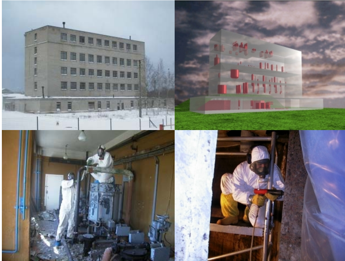
Fig. 2. The Liquid Waste Treatment Facility (LWTF)
