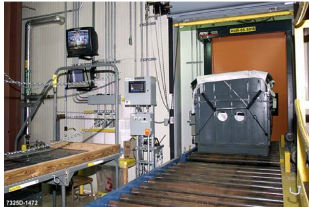
Fig. 4. The Lift-liner system is power conveyed out from loading area through a door airlock and position for final closure.
