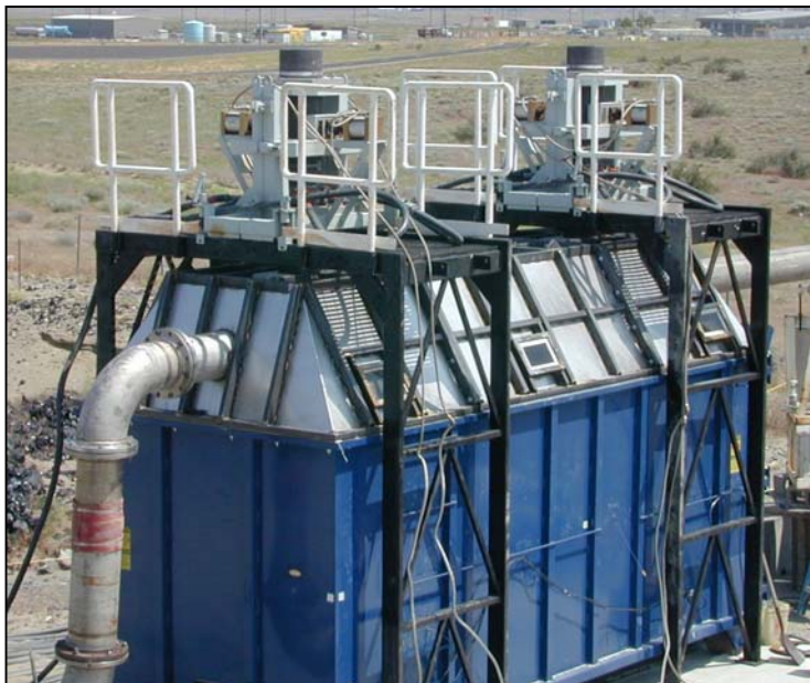
Fig. 2. Photograph of a 28-m 3 (37-yd 3 ) melt container and off-gas hood assembly during a full-scale bulk vitrification test with simulated LAW in FY-2003
