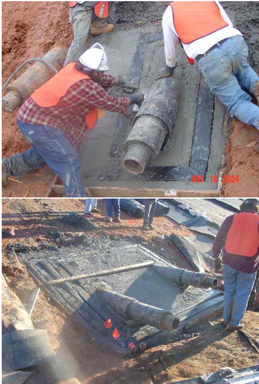
Fig. 3. Leak detection system (LDS) penetration block (top) and leachate collection system (LCS) penetration block (bottom). Details typical for both blocks.
