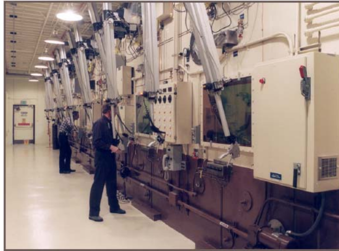
Fig. 10. Typical Hot Cell
