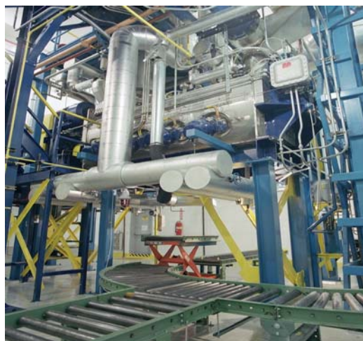
Fig. 1. Photograph of VTD unit and ancillary equipment.
