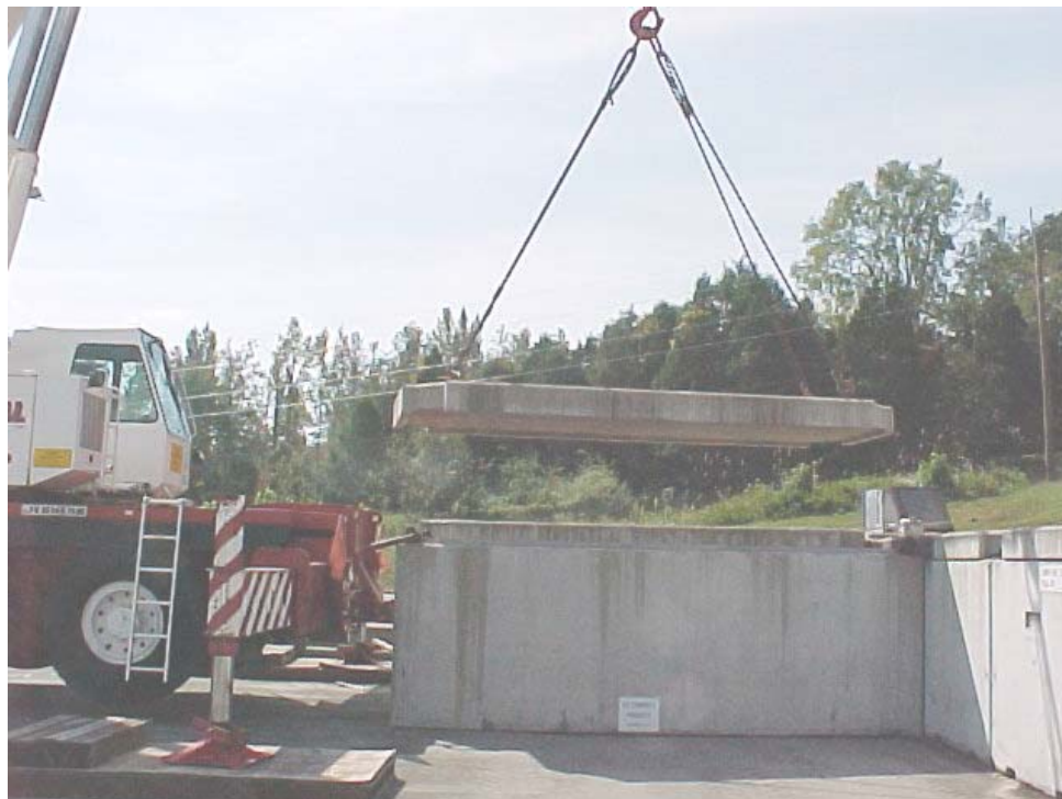
Fig. 3. A double regular vault after relocation to IWMF pad. The lid is being removed to facilitate rock-filling operations.
