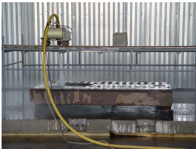
Fig. 3. A fragment of hydroabrasive cutting and decontamination of the reactor metal shielding plate
