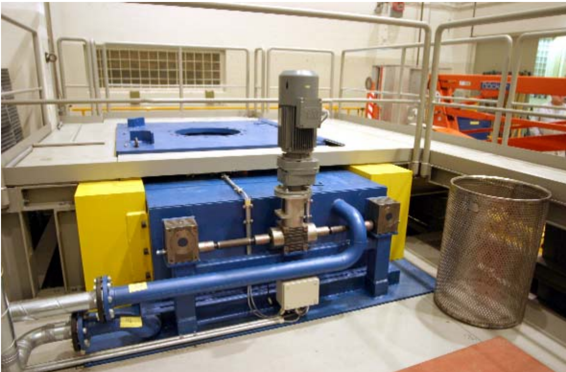
Fig. 4. Upper part of the washing plant (drum on the right)
