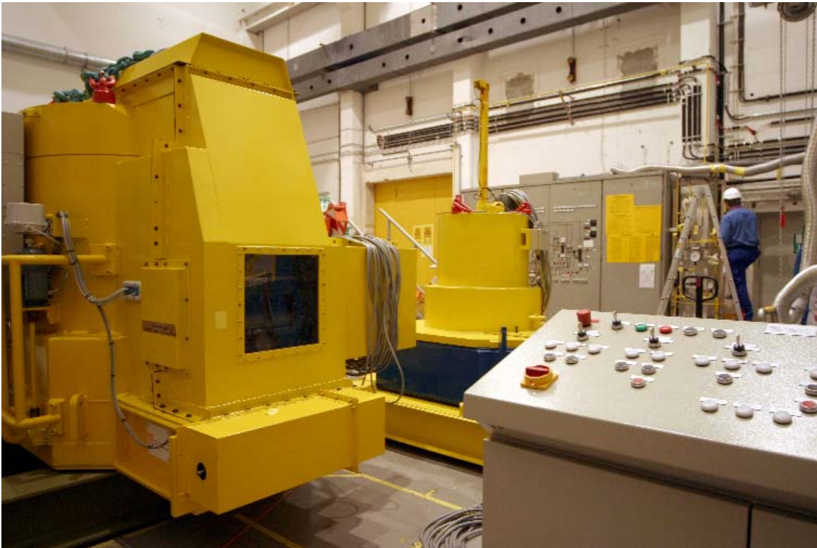
Fig. 5. Shielding bell (left) and plug removal device (back right)
