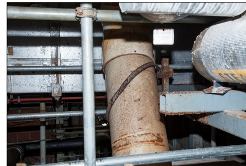
Y-12 Kathabar System Failure
