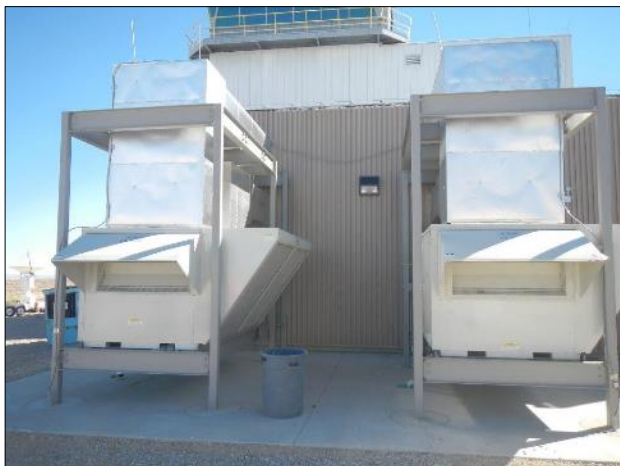
SNL Tonopah Main Distribution Hub
