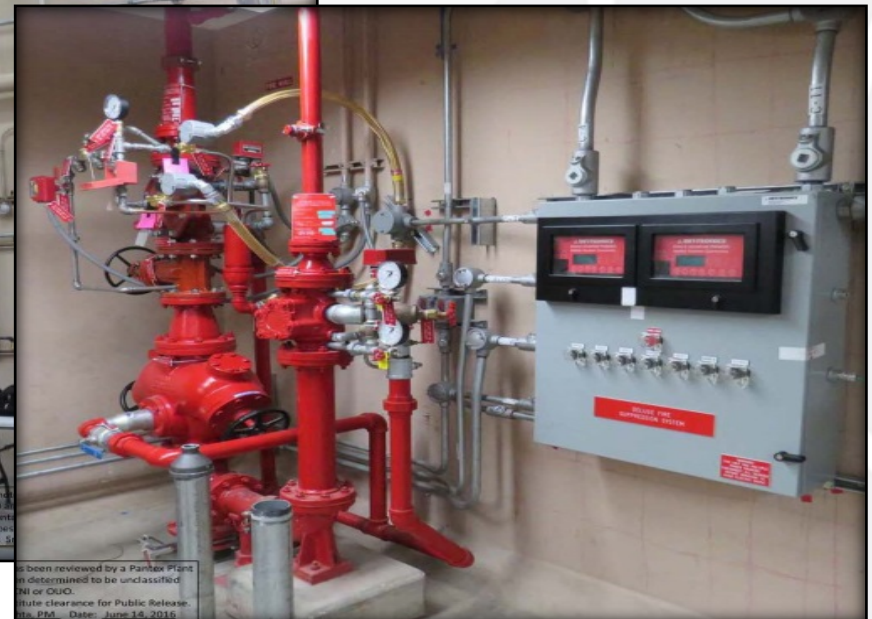
Updated control panel/riser
