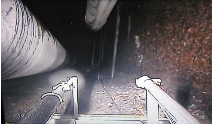
H-Canyon Air Tunnel
