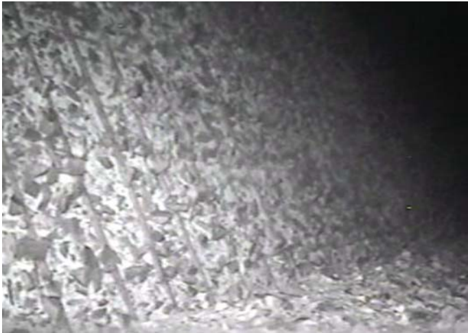
Degrading Tunnel Wall
