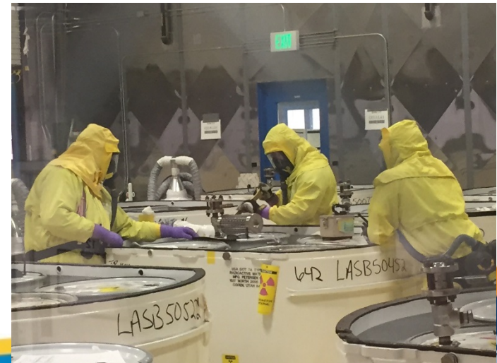
Workers installed pressure relief devices on the lids of the RNS drums
