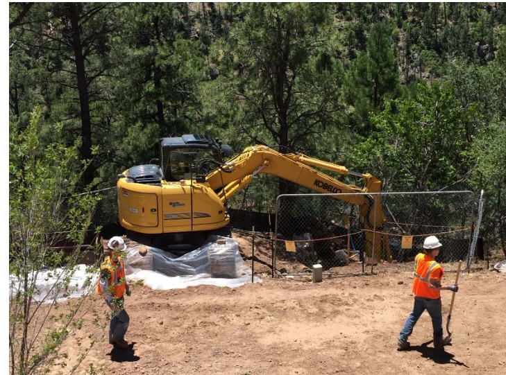
Workers used heavy equipment to remove contaminated soil from Upper Los Alamos Canyon
