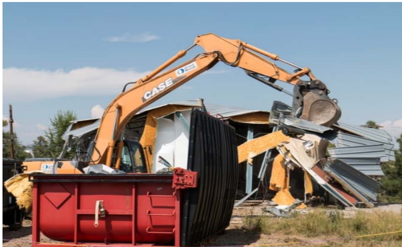
TA-21-286 was one of the last buildings at TA-21 to be demolished
