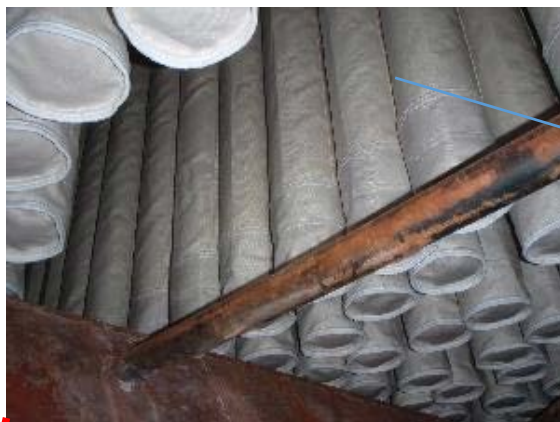
In a baghouse
