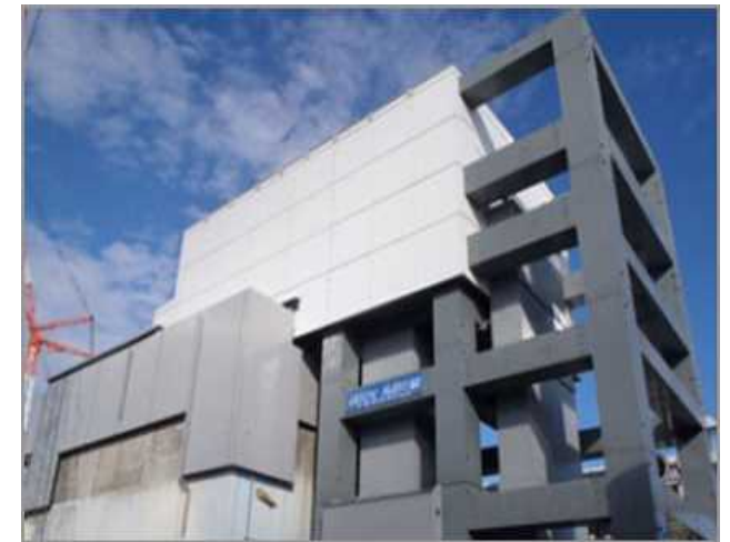
November 12, 2013: Completion of building steel framework (The volume of steel used is equivalent to those of Tokyo Tower.)
