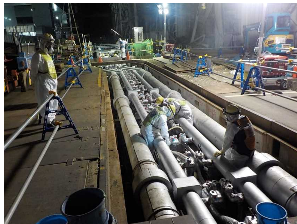
Pipe arrangement for coolant
