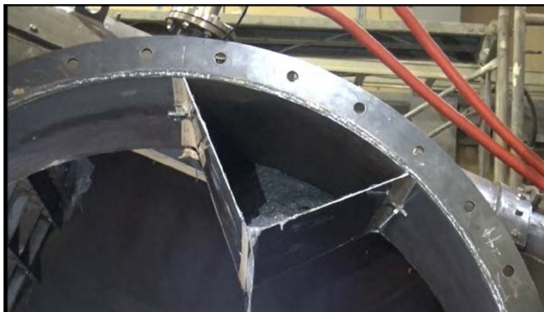
Figure 14 – V-gap plug as seen from branch.
