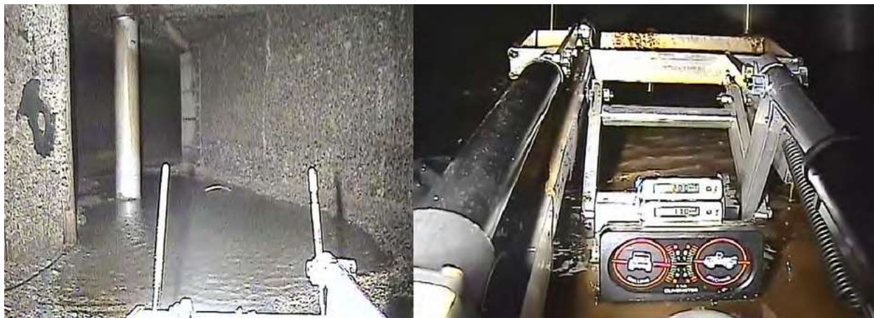
Fig. 6. Recovery Crawler in H-Canyon Air Exhaust Tunnel (CAEX) which connects the canyon to the sand filters. The RC approaches a puddle (left) and highlights the corrosion on the walls, then (right) traverses the 13-inch-deep puddle.[5]
