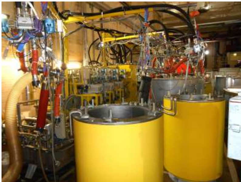
FAVORIT® installed in Circulator Hall 1
