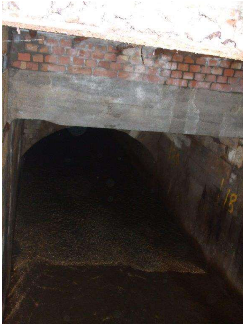
Fig. 2. Sludge Deposits in the River Race
