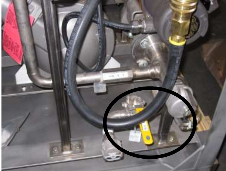
Fig.3. Potential CRUD Trap, Located just Upstream of Waste Isolation Valve (between butterfly valve and upper line)
