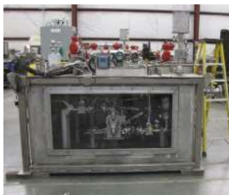
Fig. 11: Decant Pump Box at Fabrication Shop
