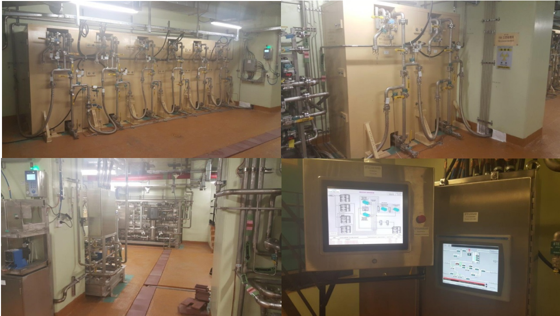
Figure 4: Yangjiang TEU after commissioning
