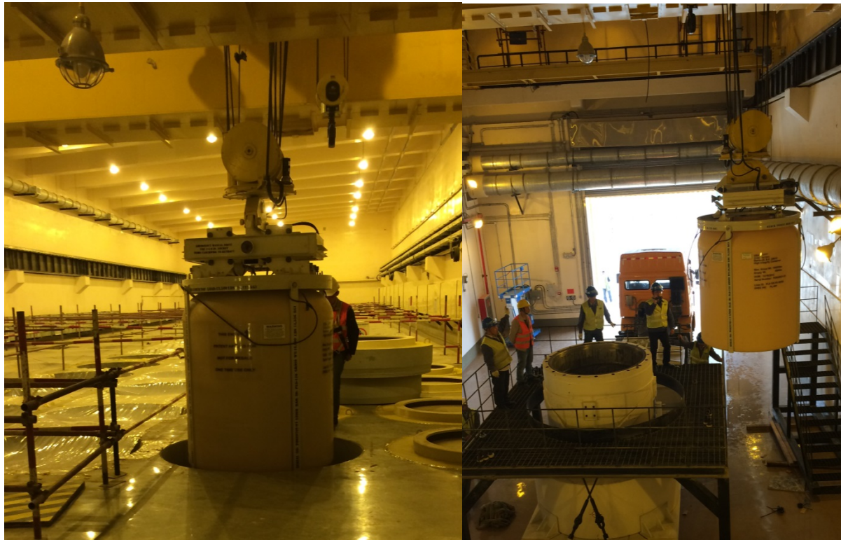
Figure 3: HIC storage area during commissioning
