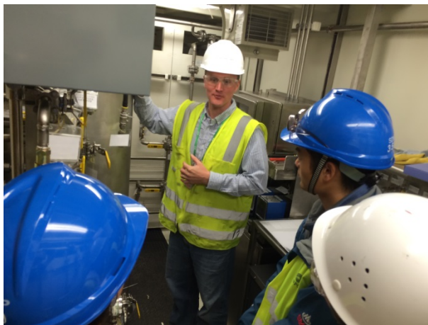
Figure 1: Mobile treatment system during commissioning
