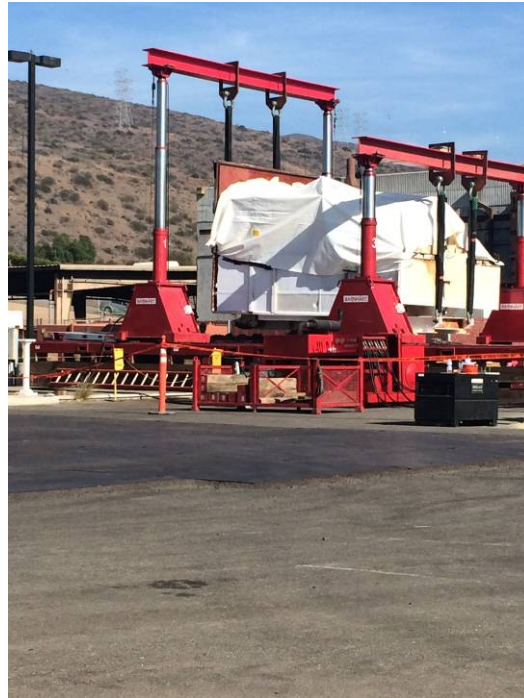
Figure 2 Down-Ending of RCP Motor #2 located in South Yard
