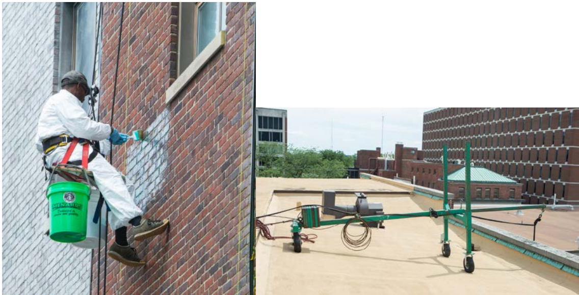
Figure 4. Bosan chair (left) and deployment from building roof (right).
