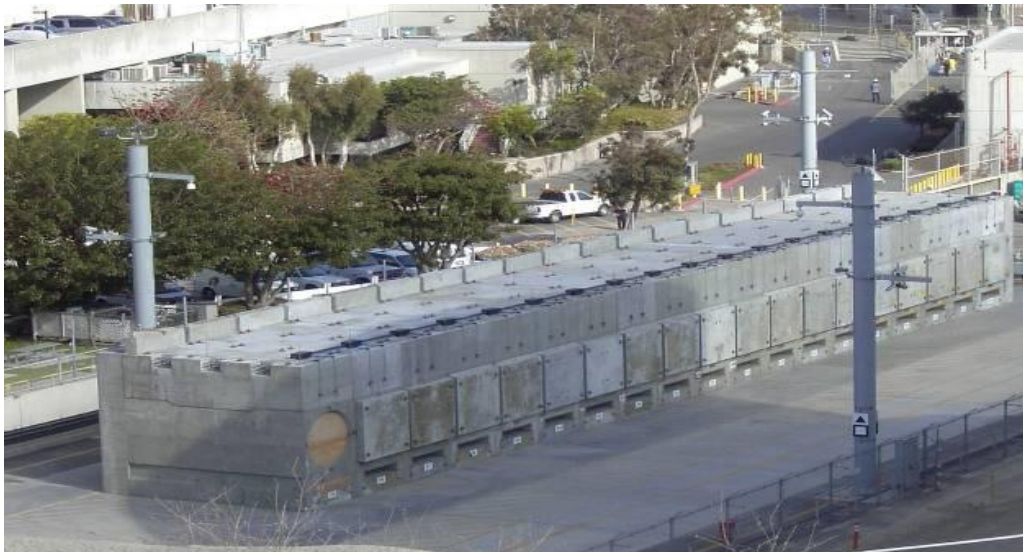
Fig.3. NUHOMS ® HSM in an array at ISFSI.
