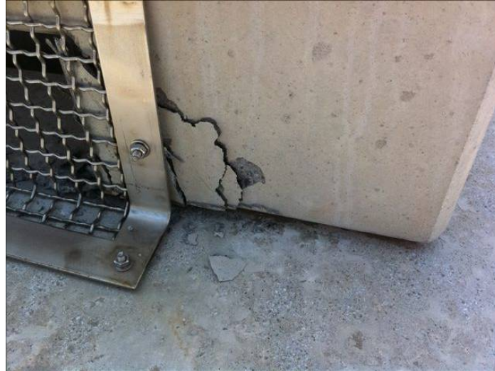
Fig. 6. Cosmetic damage to HSM after North Anna earthquake.
