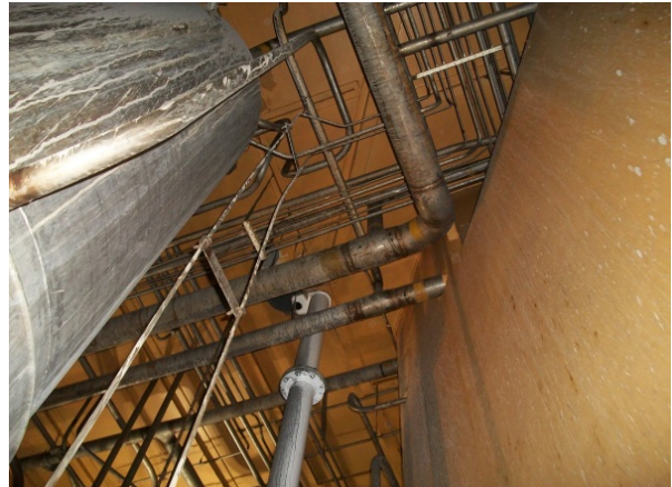
Figure 2. This in-cell photo taken before decontamination began depicts the configuration of piping and vessels in the Liquid Waste Cell.
