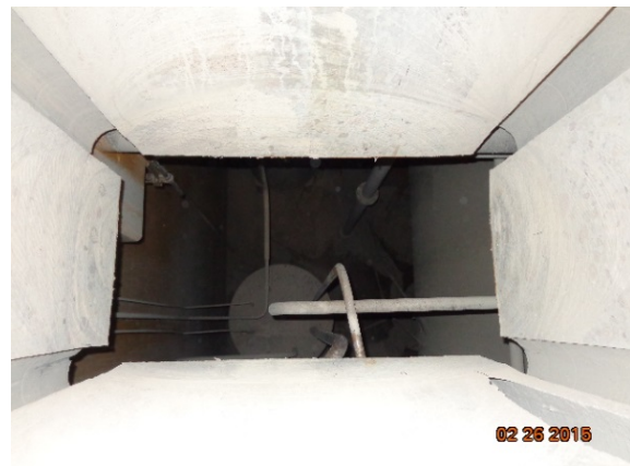
Figure 7. This is a downward view into the cell looking through a newly installed hatch.
