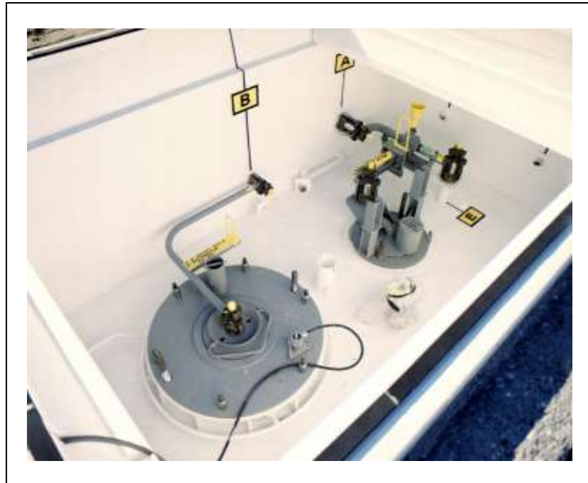
Fig. 2. Tank Farm Pump Pit with Concrete Shielding Cover Blocks Removed to Illustrate Typical Pipe Jumper Installation
