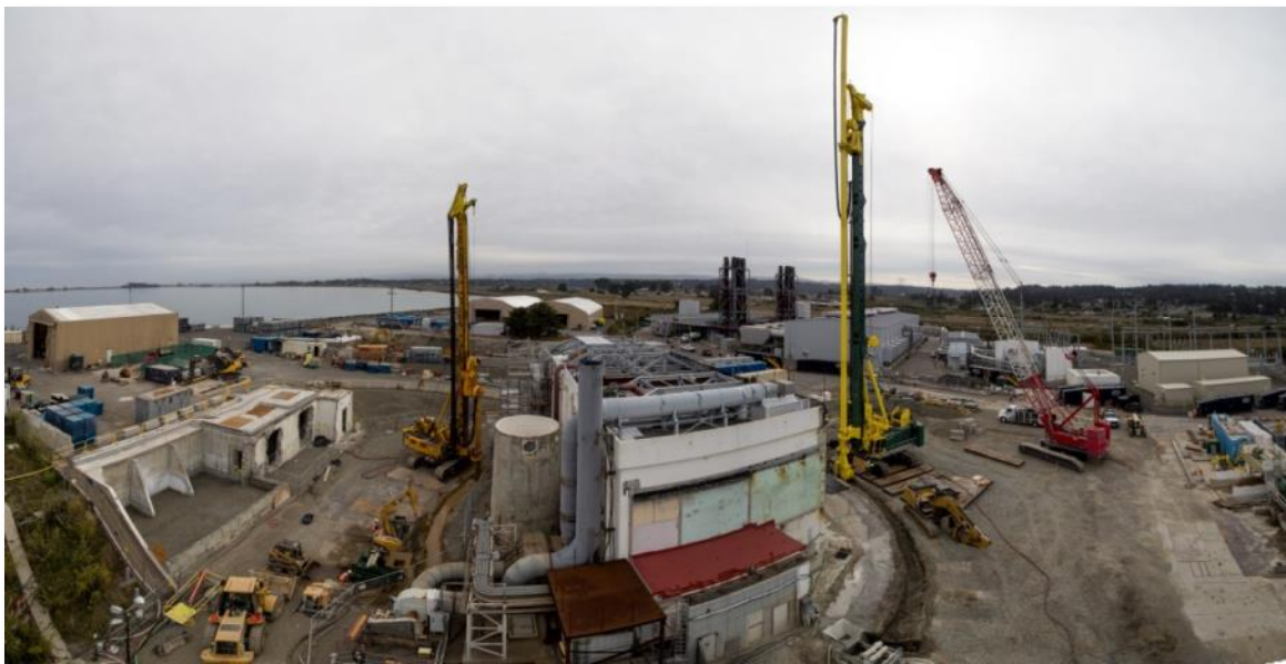
Figure 6 – CMS Operations at HBPP
