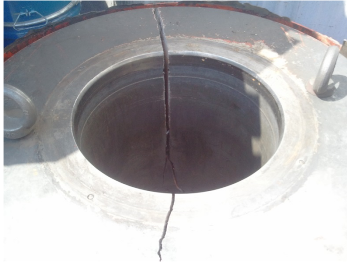
Figure 2. Through wall crack in a mono-lithic pressure vessel.
