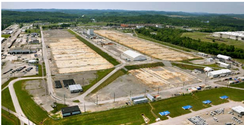
Figure 4B. The K-25 Building Pad, after Demolition (2014, with concrete slab still largely intact).
