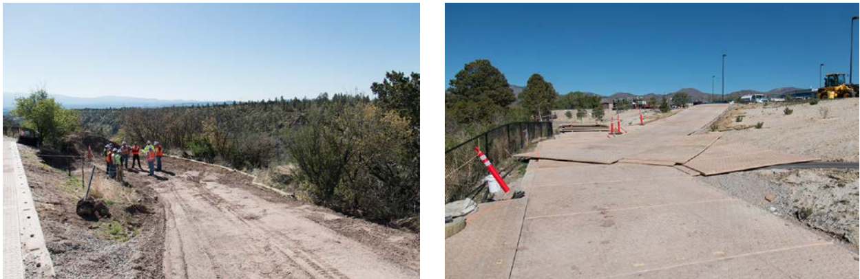
Figure 2. Lower access ramp and crane pad (left) Industrial matting over pedestrian path and upper access ramp (right). Photos courtesy of Los Alamos National Laboratory.
