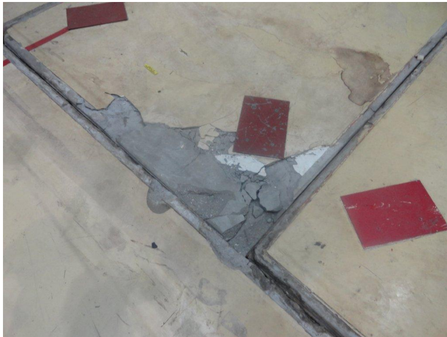
Fig. 3 – Typical concrete damage
