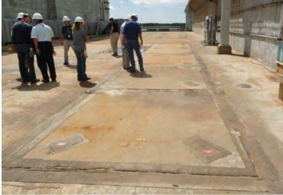
Fig. 2 Typical roof mounted access hatch with multiple shield plugs.
