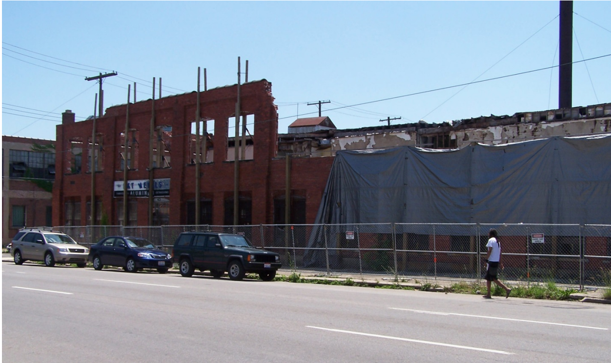
Figure 4. Columbus East, Ohio, site building in disrepair as of 2006
