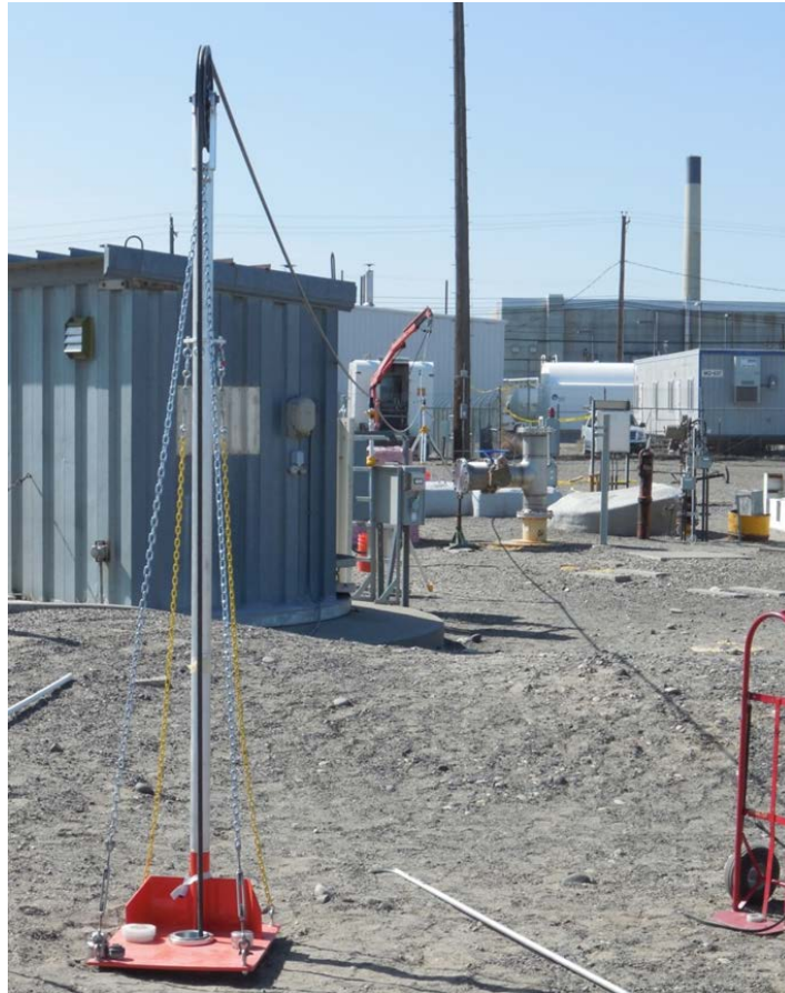
Figure 3. View of remote base, with logging cable going up and over sheave wheel with borehole probe downhole. View looking back towards logging truck. Note, this is the same setup as is shown in Figure 2.
