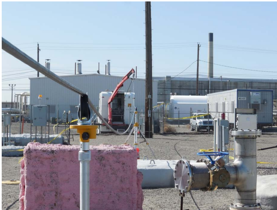
Figure 2. Intermediate cable supports shown supporting logging cable, keeping cable off of the ground. Looking back at logging truck, set up on the outside of the tank farm boundary. Note, this is the same setup as is shown in Figure 3.
