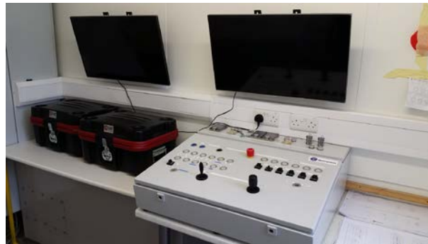
Fig. 11. ASR Control Desk
