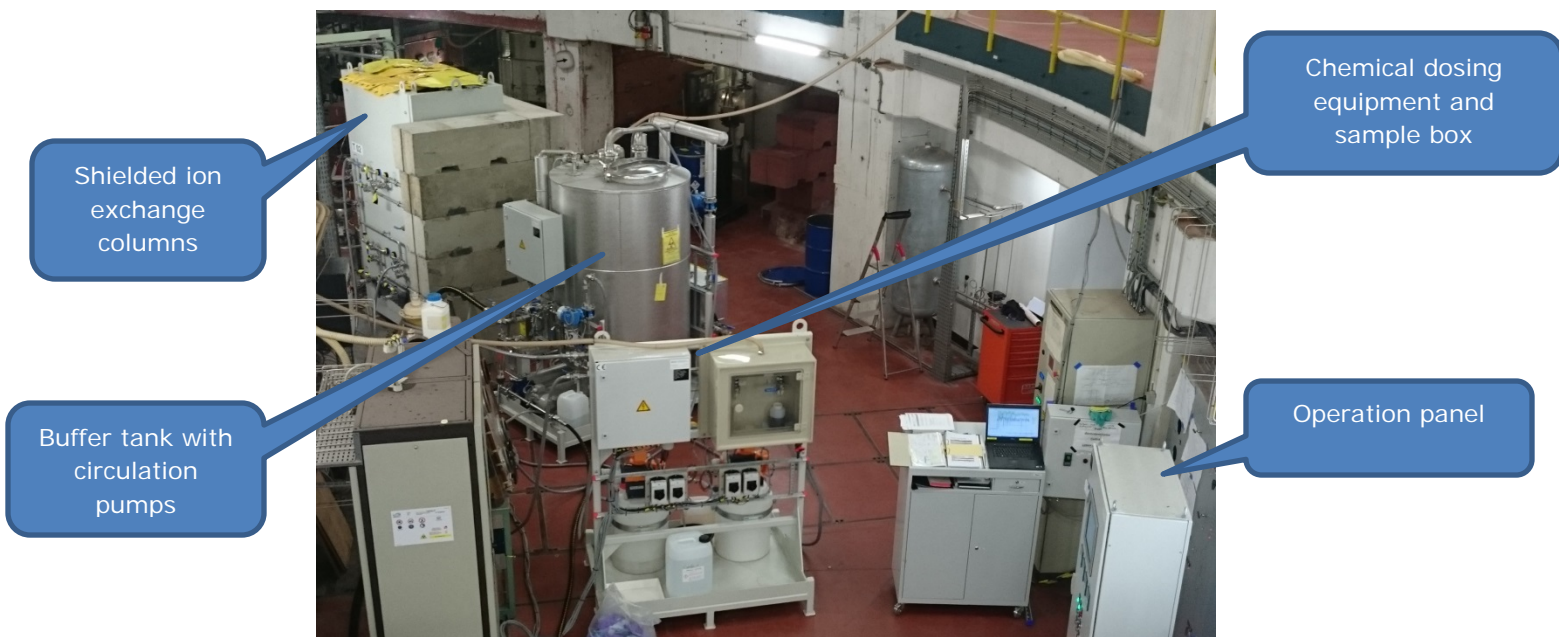
Figure 5: Installation for decontamination in the BR2 containment building
