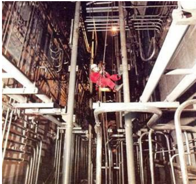
Figure 1 – Complex process cave (photo taken during commissioning)
