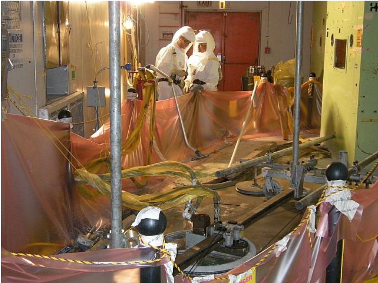
Fig. 9. A Diamond Wire Saw Being Used in the 327 Building H Cell, May 2009. It was Useful for Cutting Dissimilar Materials Including Concrete, Steel, and Heavy and Light Gauge Materials.
