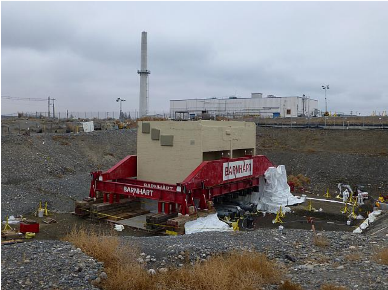
Fig. 12. The 340 Vault is Prepared to be Lifted and Transported to ERDF for Disposal, January 2014. The Vault had a Lift Weight of 2.3 Million Pounds and a Transport Weight of 3 Million Pounds.
