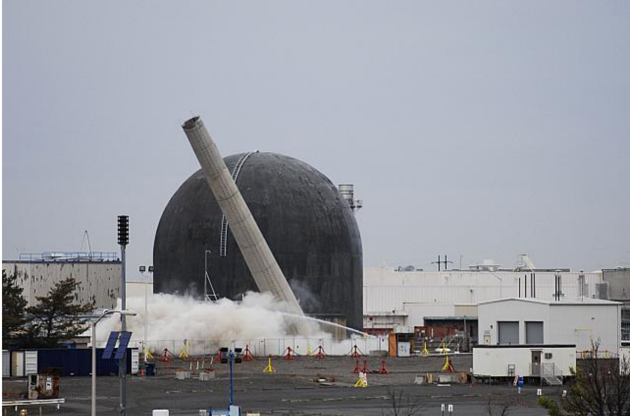
Fig. 6. The 309 Stack is Brought Down by Explosive Demolition in the 300 Area, October 2010.
