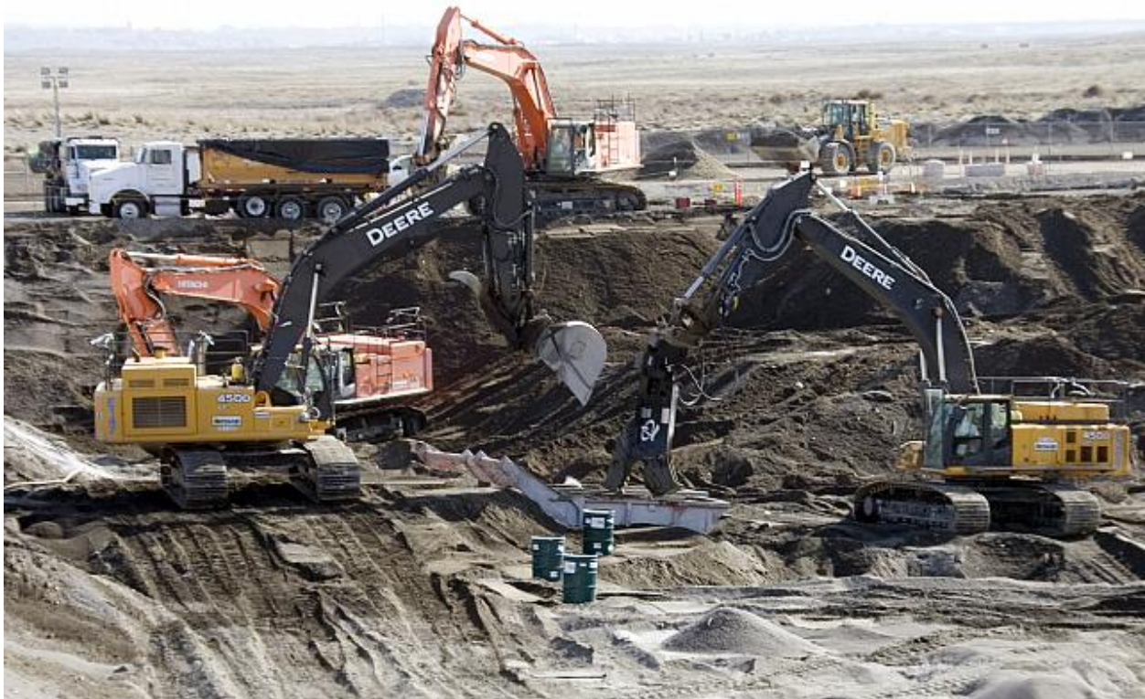
Fig. 2. Waste is Excavated, Placed in Drums, and Processed at a 618-10 Burial Ground Trench, March 2015.
